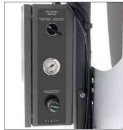
Control board for media tensioning
